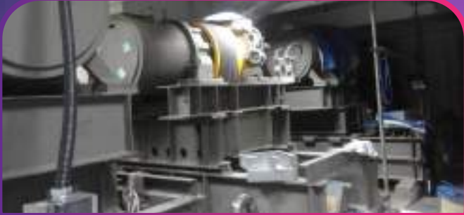
Lotus Tower CCTV
